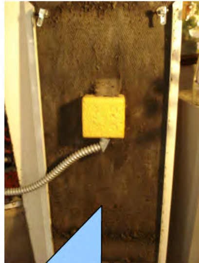
Dust lint build-up on back of HVAC panel
